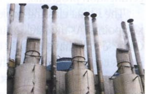
Water scrubber system
